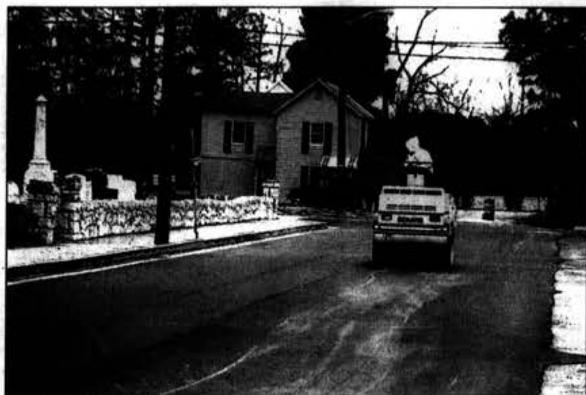
Antioch Avenue in Princess Anne is paved last week as the months of Streetscape construction nears an end. Work should be completed sometime this month.
